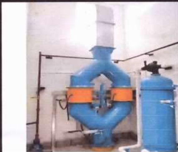
Ventilation System to remove noxious gases produced in irradiation cell during process like Ozone, CO, CO 2
