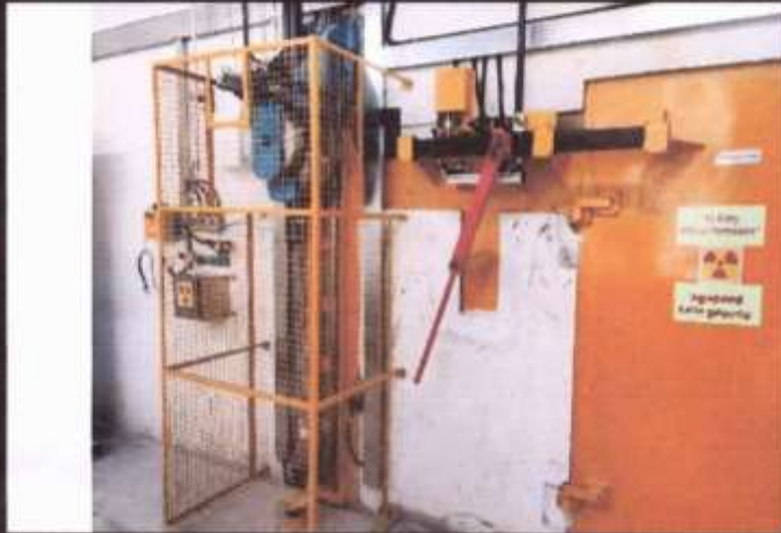
Safety control Systems
