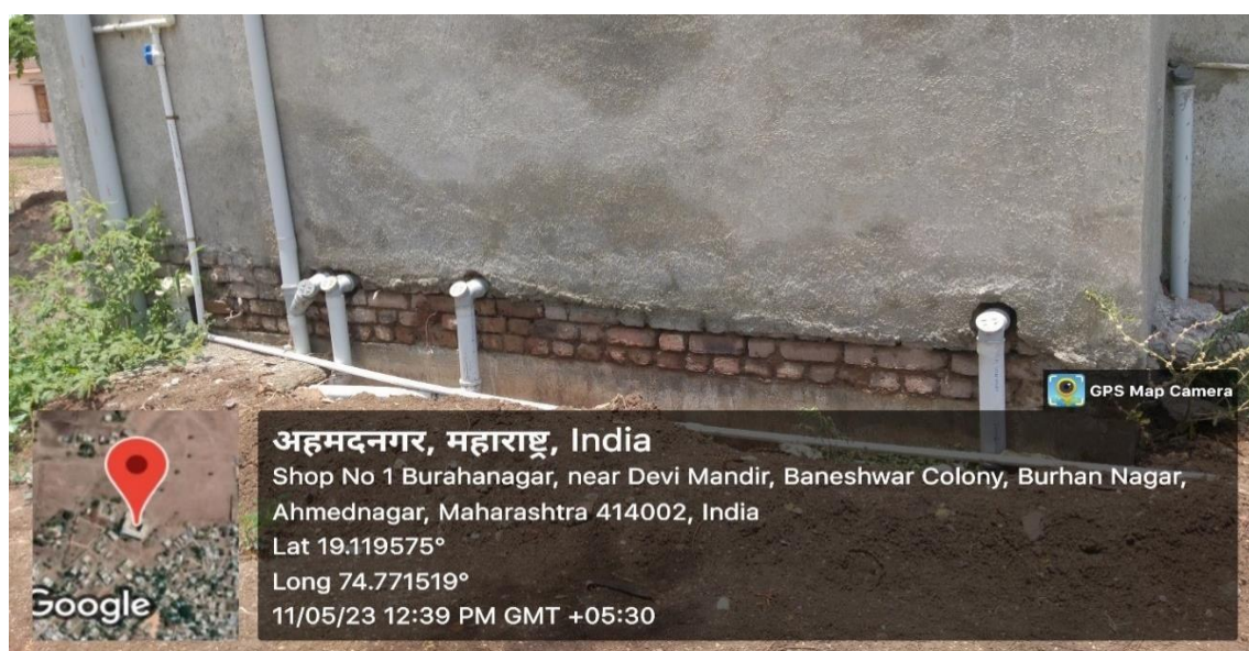
Liquid Waste Soak Pit
