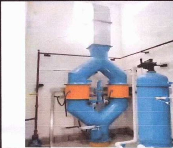
Ventilation System to remove noxious gases produced in irradiation cell during process like Ozone, CO, CO 2
